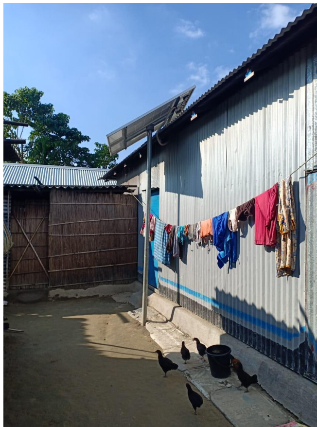
Image s. An SPV Standalone Solar Panel in the char
