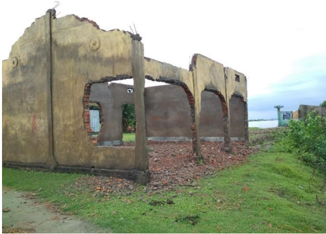
Image d. The destroyed LP school at Ramapara Pam char.
