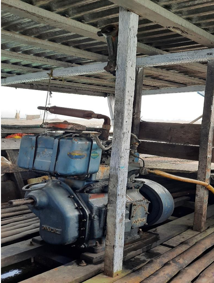
Image i. The diesel engine, taking up a lot of space inside the ferry.
