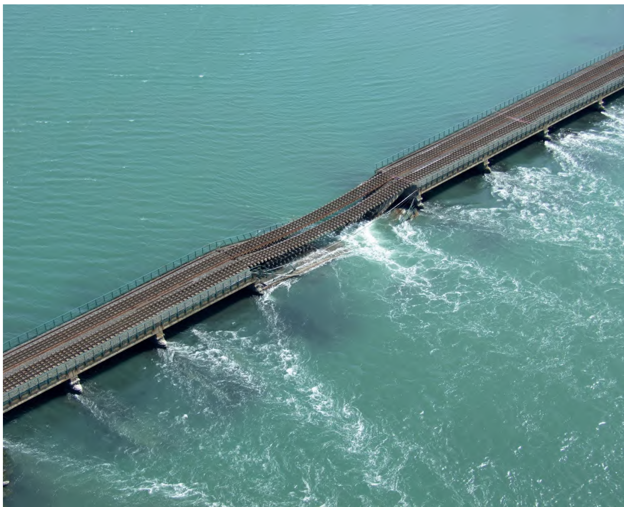
Figure 7.1 Aerial image of the section of the Broadmeadow viaduct near Malahide that collapsed on 21 August 2009. Source: https://cdn.ca.emap.com/wp-content/uploads/sites/9/2009/09/0908230099.jpg
