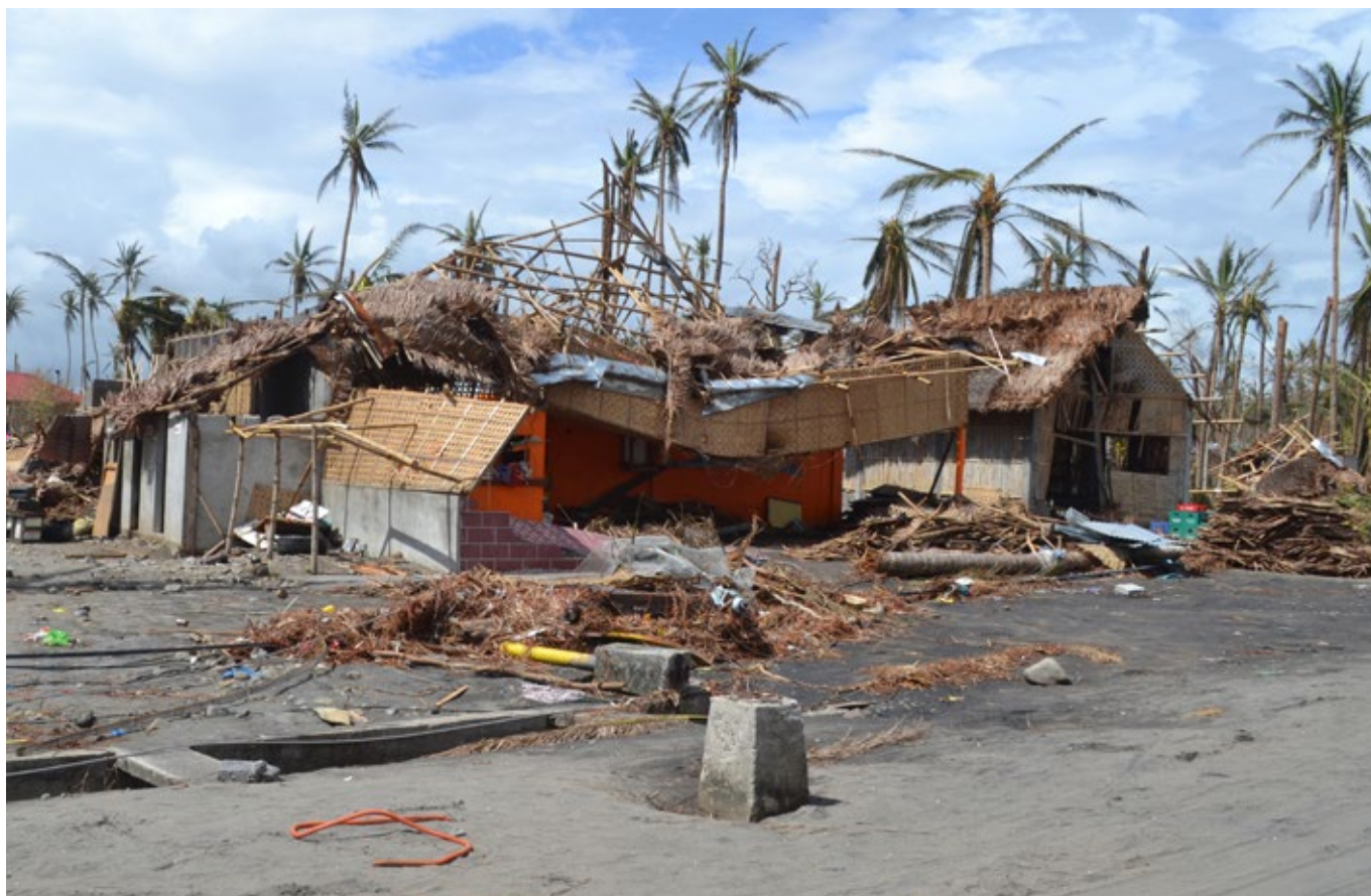
A destroyed house on the outskirts of Tacloban on Leyte island. This region was the worst affected by the typhoon, causing widespread damage and loss of life. Caritas is responding by distributing food, shelter, hygiene kits and cooking utensils.
