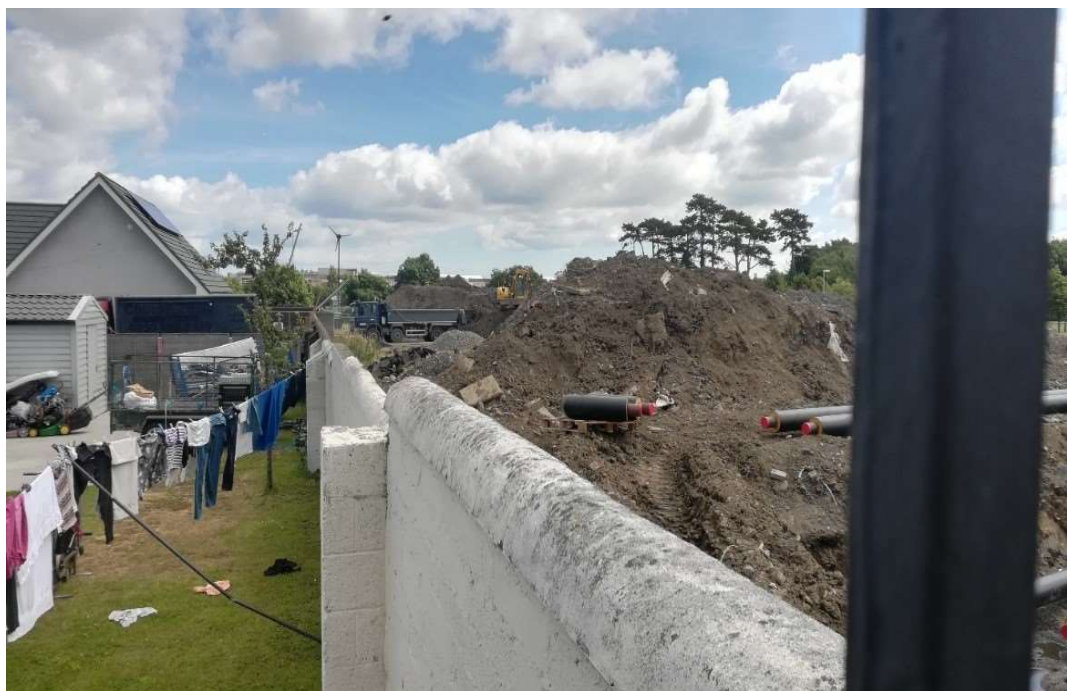
Plate 5.11: The district heating pipe works (right) adjacent to the Traveller residential estate (left) (Source: Author, 2021)
