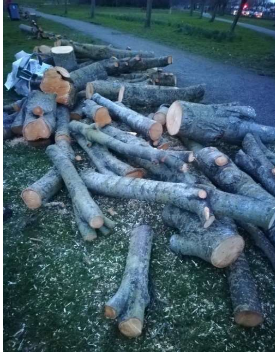
Plate 4.8: Tree removal in Tymon Park South as part of the planned flood works (Source: Author, 2024)
