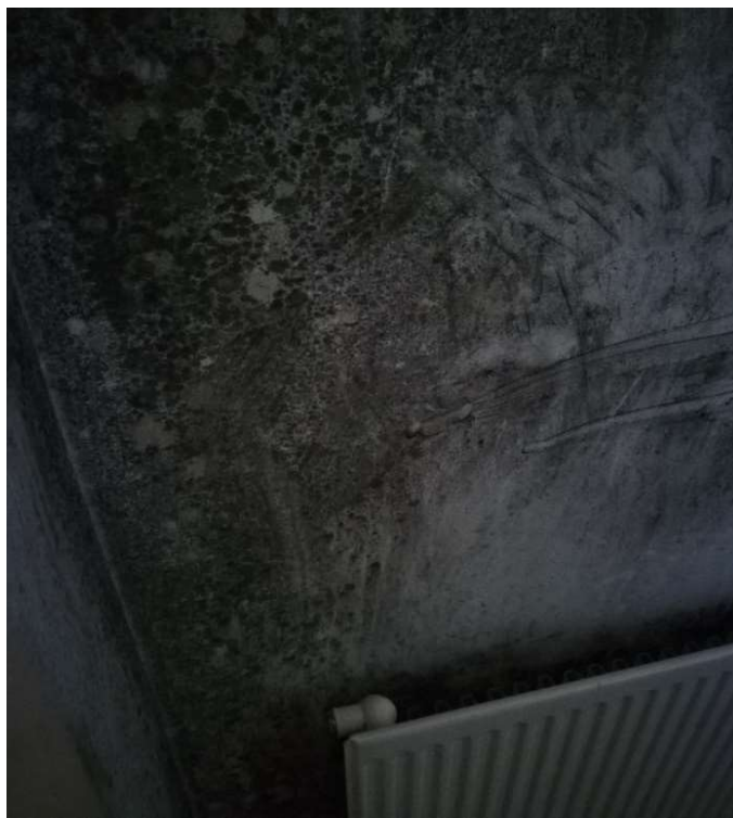
Plate 6.12: Walls covered with mould in Dublin City Council managed flats adjacent to the Guinness factory site and Storehouse (Source: Author, 2023)
