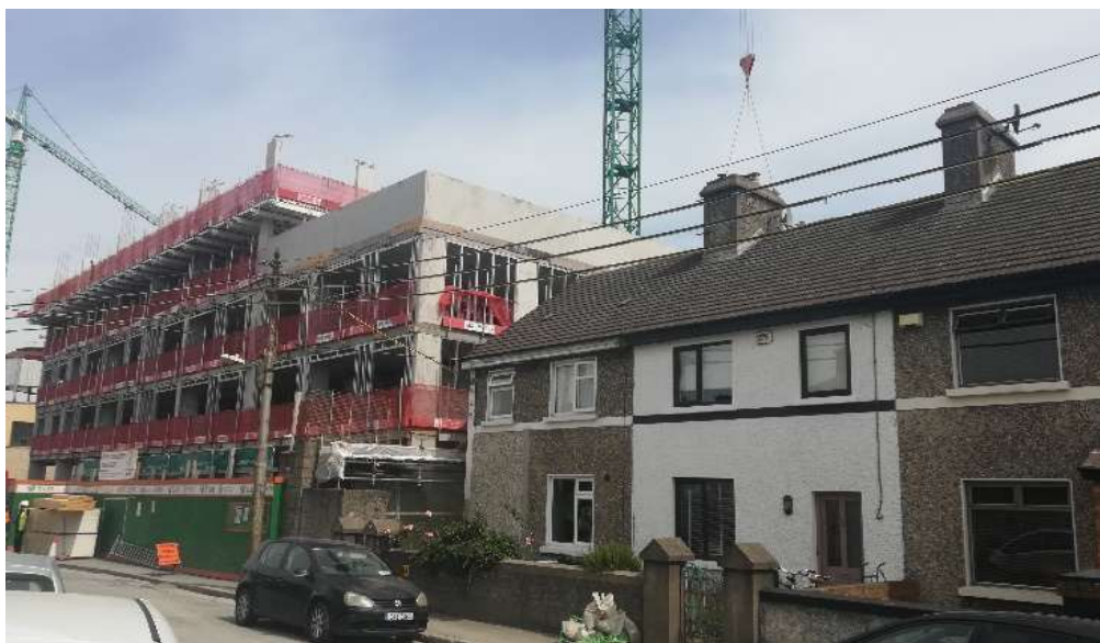
Plate 6.2: GSA/Creedon Group BTR and SA construction works on the side of existing houses (Source: Author, 2021)
