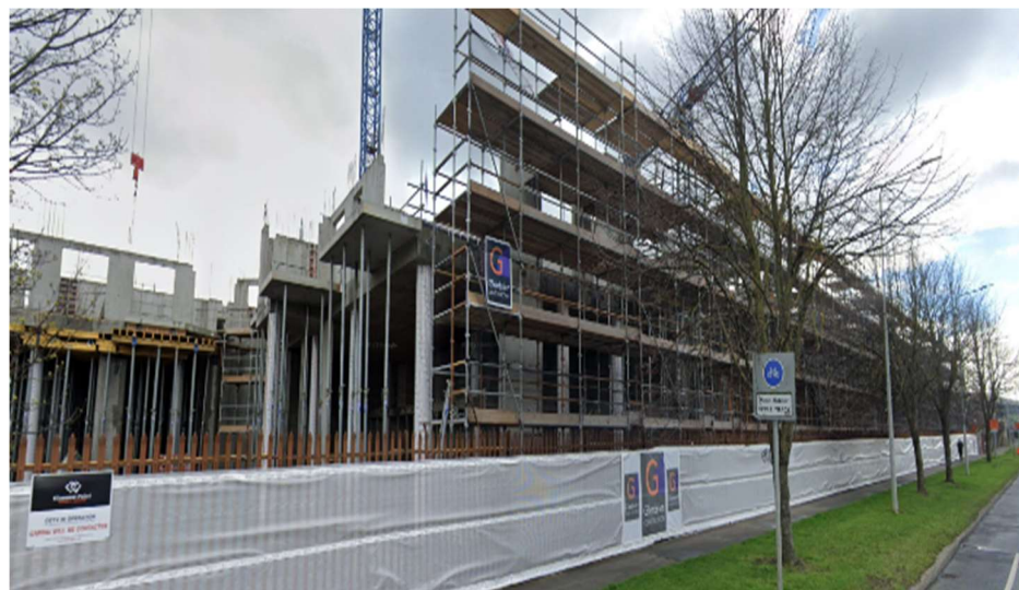
Plate 5.7: Build-to-rent development erected on the culverted Poddle mapped as a 1050mm surface water drain in the planning application (Source: Google Maps, 2023)
