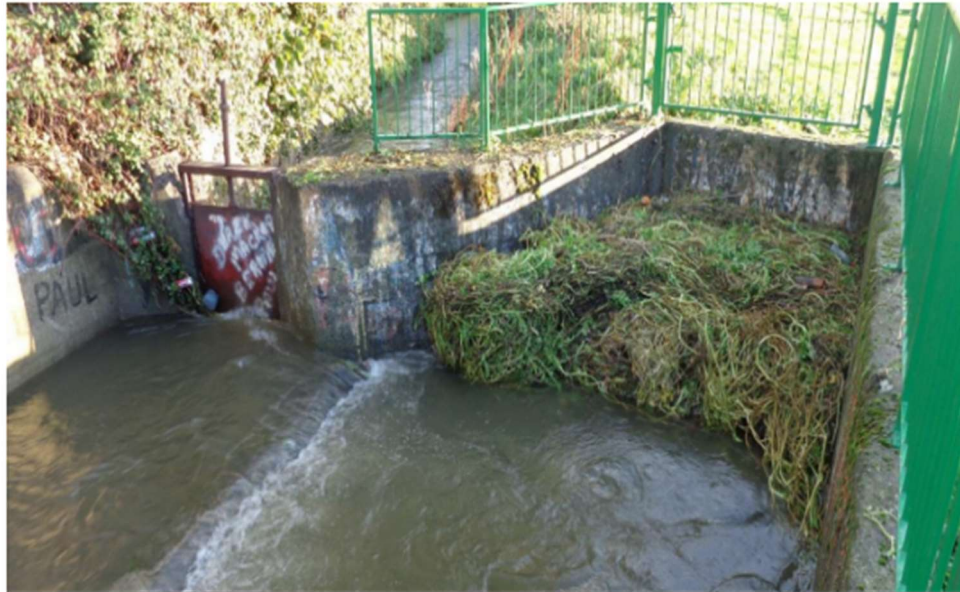
Plate 4.3: River Poddle overflow culvert blocked by vegetation in Wainsfort Manor (Source: Waterman Moylan Consulting Engineers Limited, 2016)
