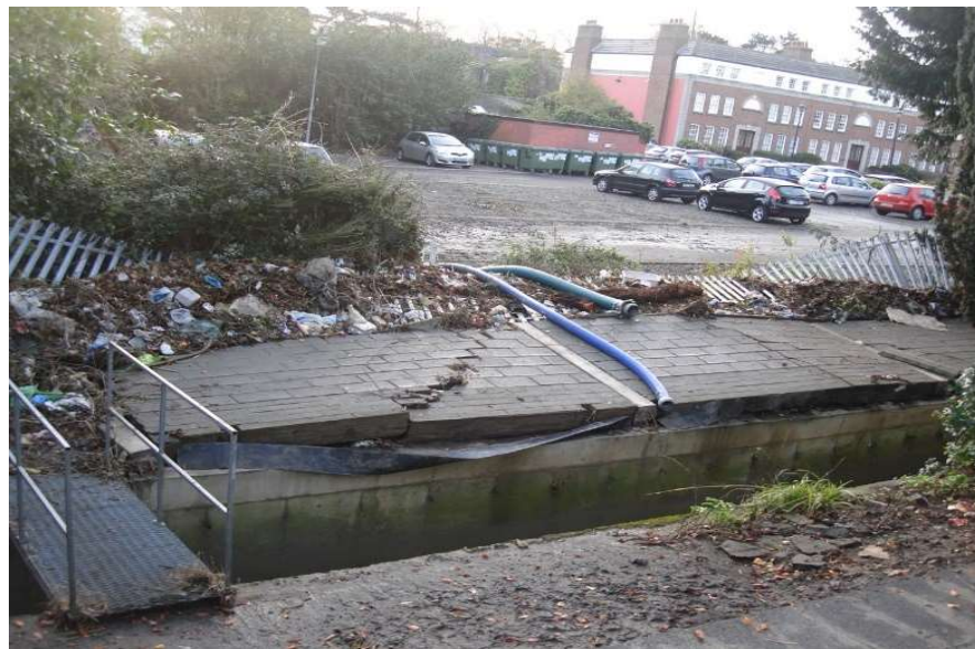
Plate 4.2: Photograph of the Gandon Close wall after the 2011 flood event (Source: Dublin City Council, 2019c)
