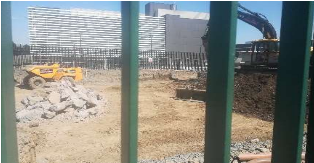
Plate 5.5: The former site of the social club during the new district heating energy centre construction works (Source: Author, 2021)
