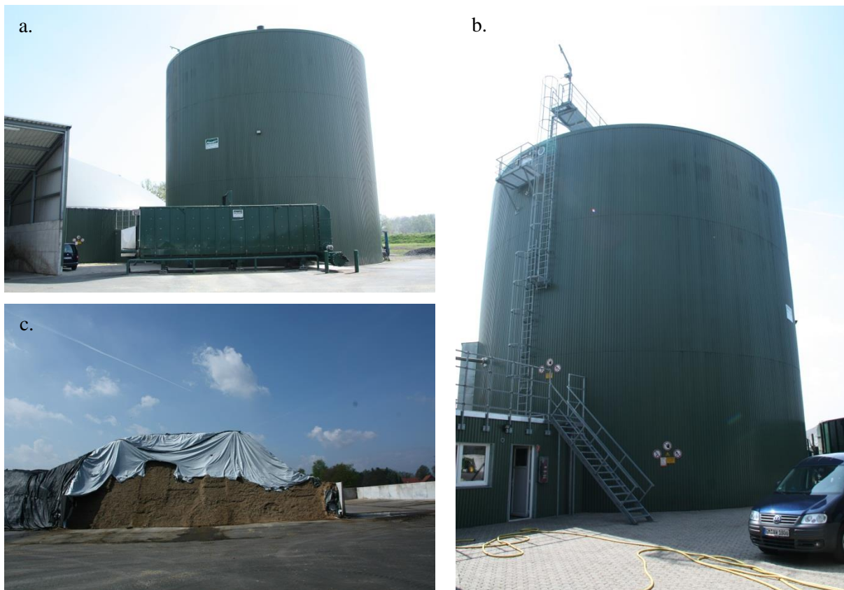
Figure 3-3: Sunderhook ABP - a. primary digester with system for solid substrate input, b. primary digester, c. drive-in silo for maize and rye
