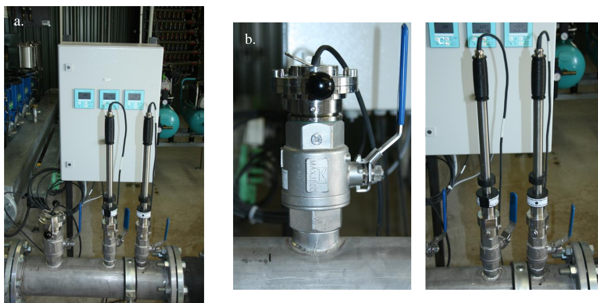
Figure 6-12: Installation of pH, ORP and TS probe at the Sunderhook ABP: a. complete installation, b. TS probe, c. pH and ORP probe
