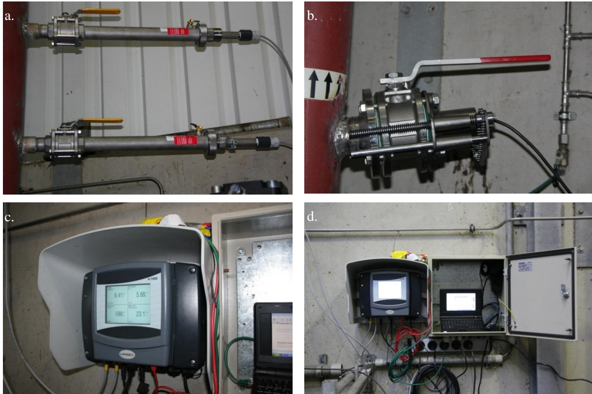
Figure 6-22: Installation of the probes at Industrial I. a. pH and ORP probes, b. TS probe, c. SC1000 controller, d. Overview of probe control and data acquisition
