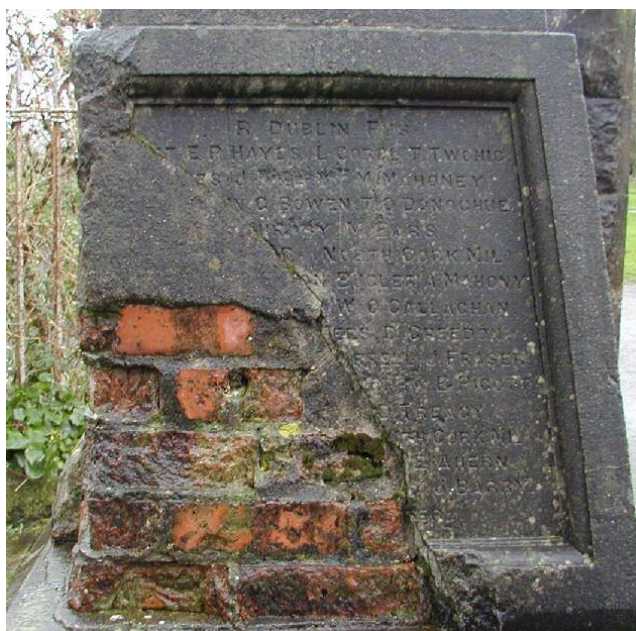
Fig. 65: A contemporary photograph of the damage caused by the explosion at the South African War memorial in Connaught Avenue, Cork (2014)
