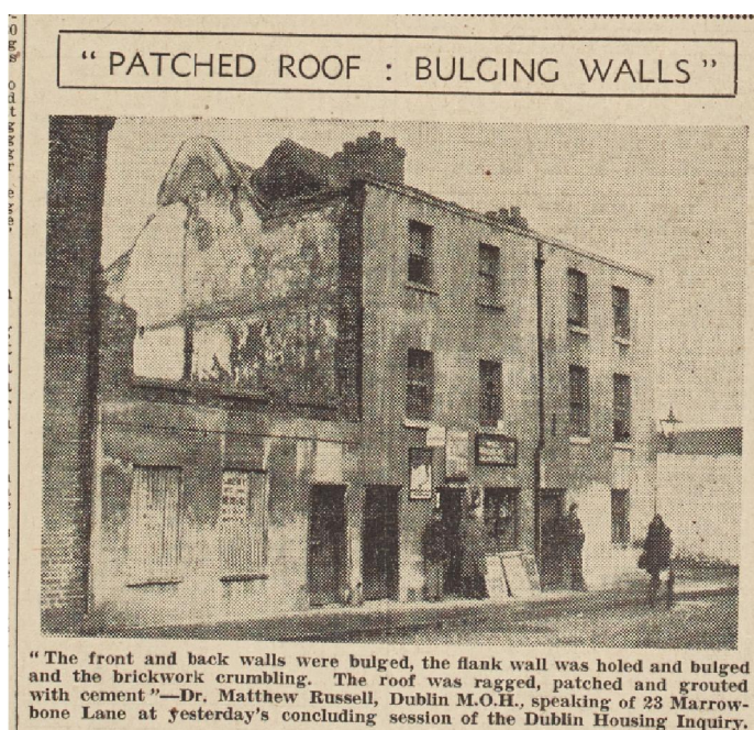
Figure 16 Patched Roof Bulging Walls. Image Courtesy of the National Library of Ireland.
