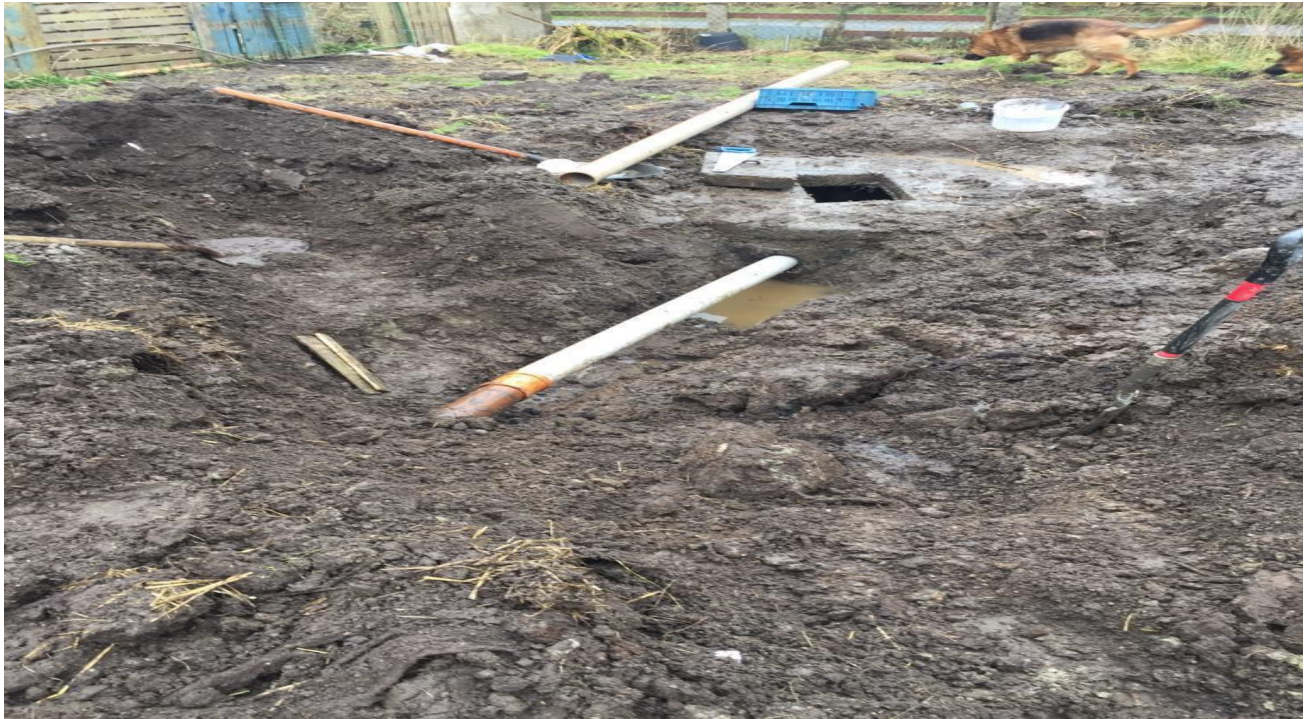
Figure 19 Septic tank issues
