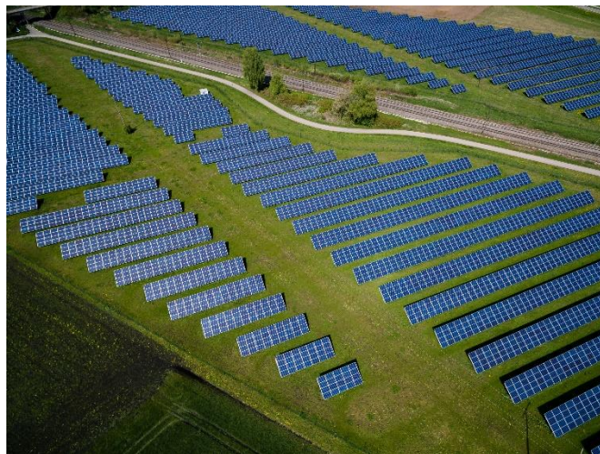
Figure 4. Ground mounted PV arrays (credit: andreas-gucklhorn-llpf2eUPpUE-unsplash)
