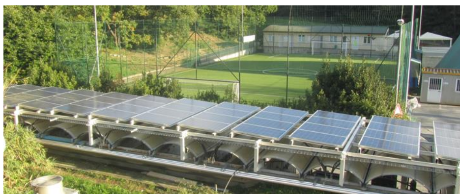
Figure 21. Integrated photovoltaic/Thermal (PV/T) collectors (PV/SAHP system). University of Genoa Campus, Italy
