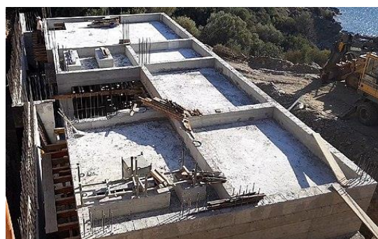
Figure 33. Construction of an extensive green roof in Likorema (Euboea, Greece) (Etan J. Tal, CC BY-SA 4.0, via Wikimedia Commons)
