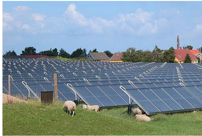
Figure 22. District heating by a solar thermal collector field of 18300 m 2 . Marstal, Denmark (credit: Erik Christensen, CC BY-SA 3.0 < https://creativecommons.org/licenses/by-sa/3.0/ >, via Wikimedia Commons)
