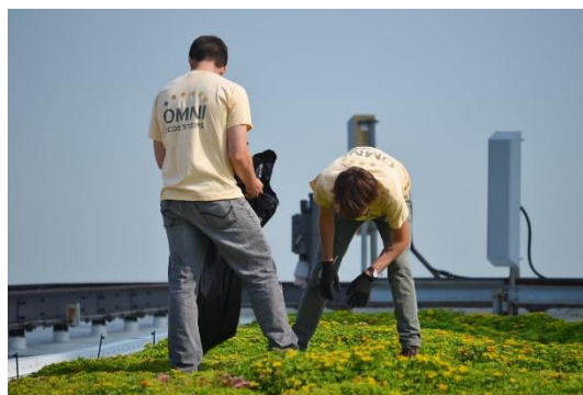
Figure 36. AMA Plaza (Chicago) Green Roof Maintenance (credit: Flickr, Attribution-ShareAlike 2.0 Generic, CC BY-SA 2.0)
