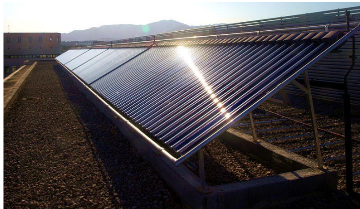
Figure 13. On roof thermal collector system for DHW (credit: Chixoy, CC BY-SA 3.0 < http://creativecommons.org/licenses/by-sa/3.0/ >, via Wikimedia Commons)
