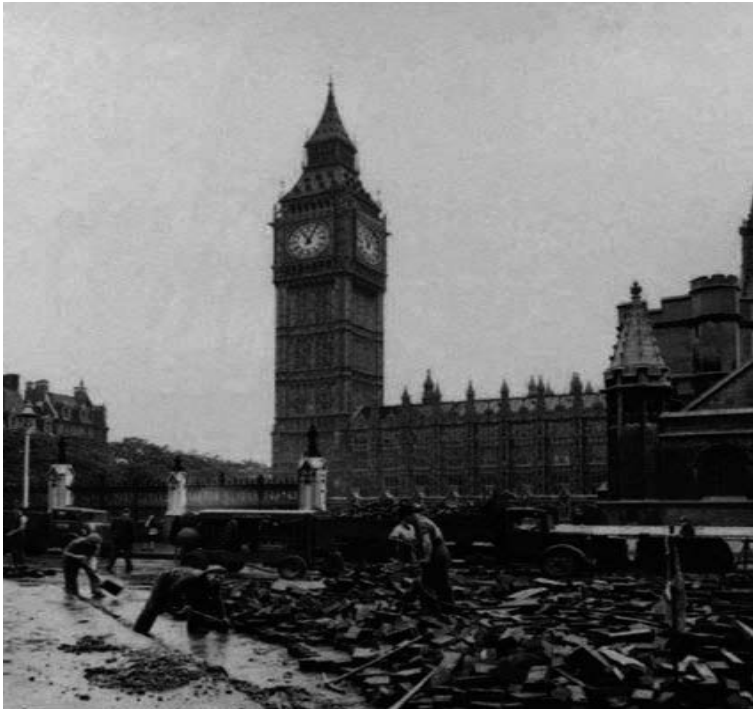
Figure 5 - Fitzpatrick labour – mostly Irish migrants - reconstructing Parliament Square, London, probably c.1930s. (Photo source: Volker-Fitzpatrick PLC)
