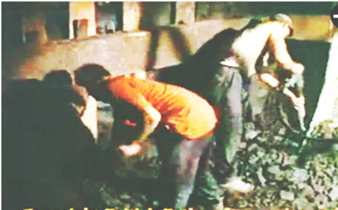
Figure 3.9 - Irish 'tunnel tigers' – almost certainly Donegal men - working with pneumatic airspades at tunnel face.
