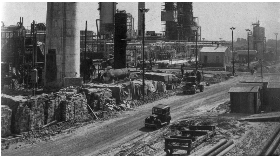
EUROPE'S LARGEST OIL REFINERY—PROGRESS ON THE ESSO REFINERY AT FAWLEY, HAMPSHIRE, WHICH IS TO GO INTO PRODUCTION IN THE AUTUMN : A view of the distillation units at the refinery which is being constructed by the Esso Petroleum Company (lately Anglo-American Oil Co.) on the shores of Southampton Water. Rising in the foreground is the chimney-stack of the boiler-house. Inset above on right—Construction work in progress on a 49-ft.-diameter sphere which will be used for the storing of butane.
