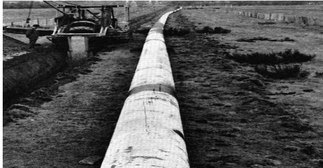
Figure 4 - High-pressure gas mains installation being undertaken by J Murphy & Sons Ltd in 1960s. (Source: 60 Years of Defining Moments: A History of Murphy , (London, 2011), p.16)
