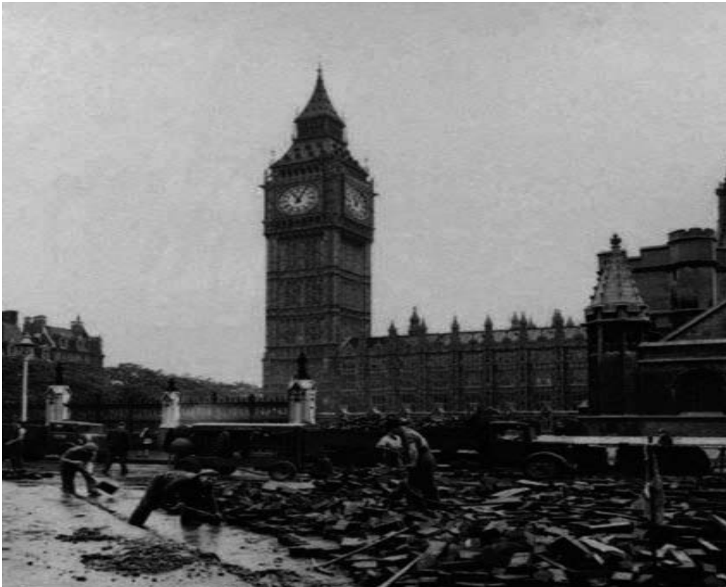
Figure 3.2 - Fitzpatrick & Sons Ltd labour repaving Parliament Square, c.1924 (Source: Volker Fitzpatrick PLC website, available at http://www.volkerfitzpatrick.co.uk/en/aboutus/storysofar [accessed March, 2015])
