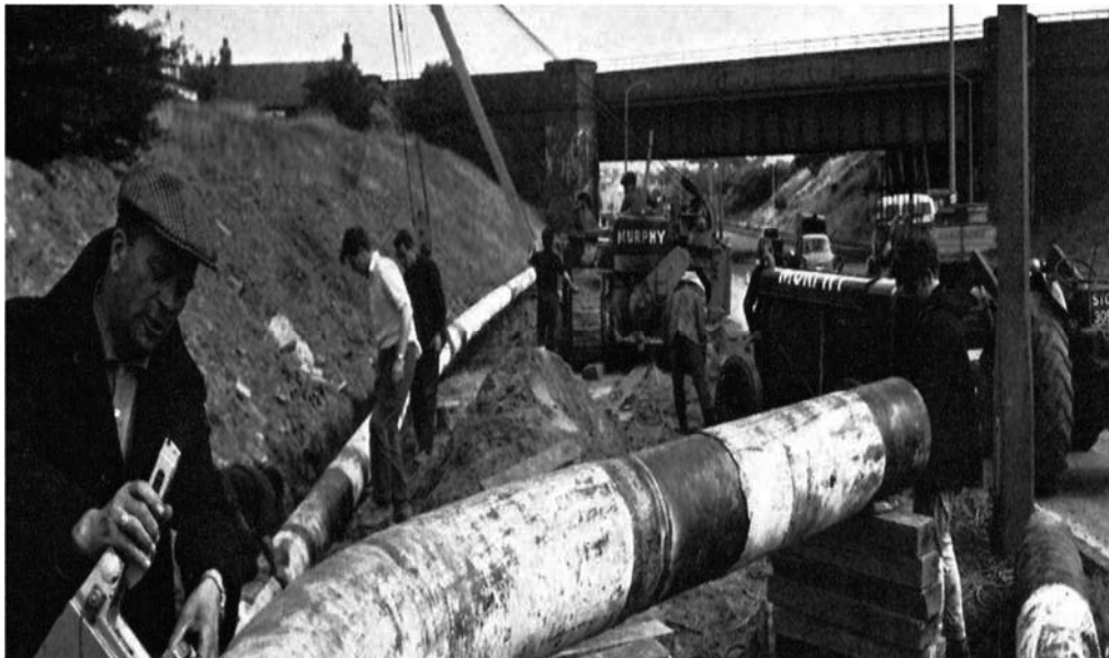
Figure 3.12 - - Irish migrant labour working for J Murphy & Sons on high-pressure 'trunk' gas mains and sub-mains for North Thames Gas Board in mid-1960s
