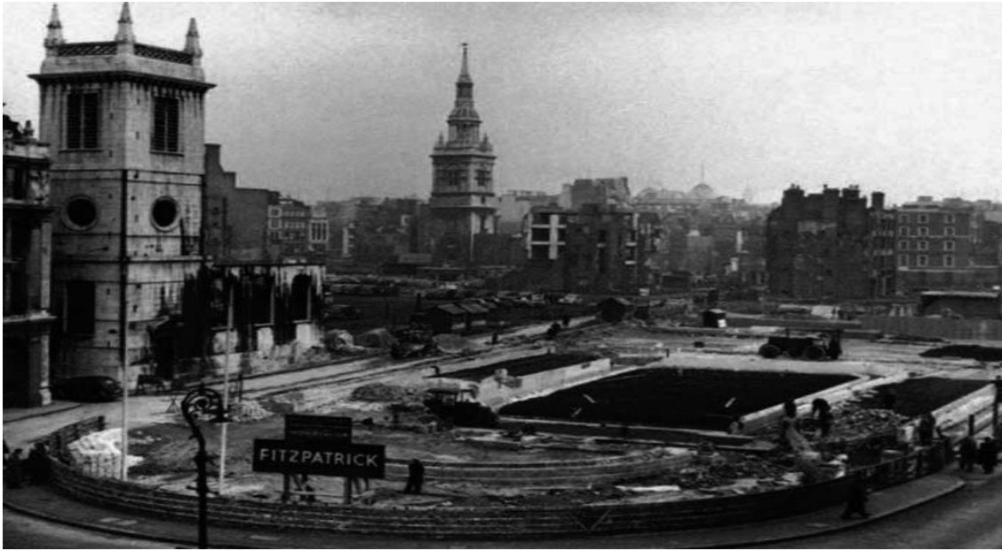
Figure 6 - Fitzpatrick & Sons Ltd - refurbishment of Parliament Square, London, c1930s (photo: courtesy of Volker-Fitzpatrick PLC)
