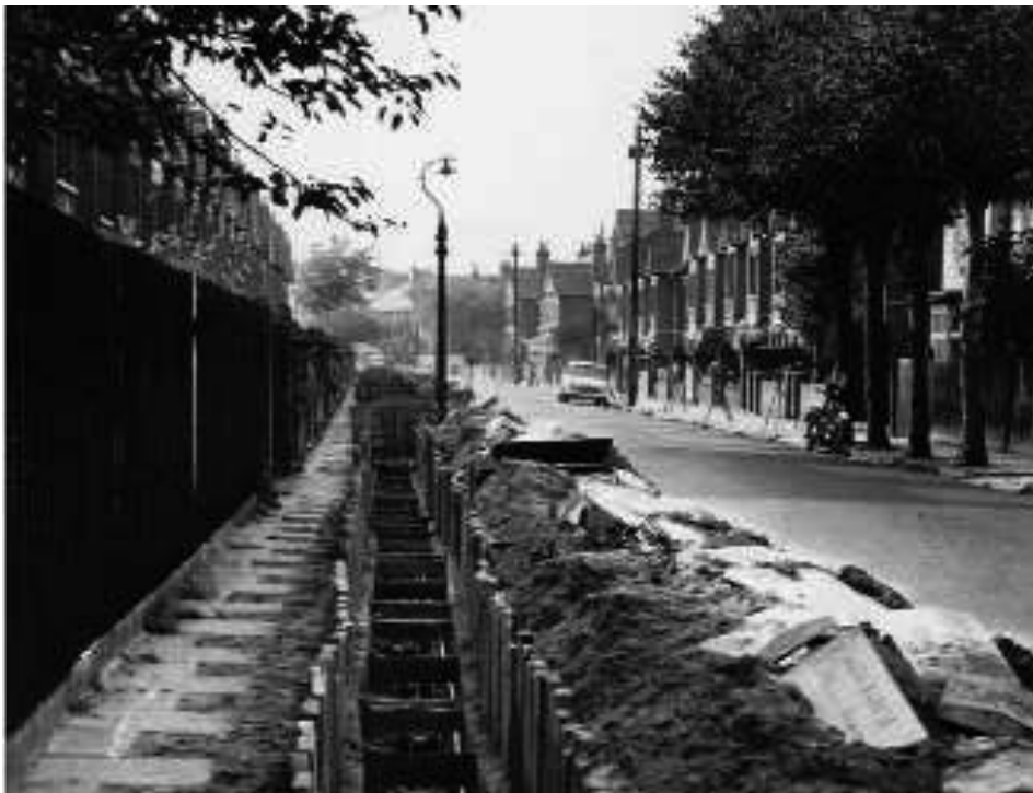
Figure 4.9 – Typical London infrastructure gas/cable installation trench from late 1950s - showing earthwork support in place (Source: http://www.lowery.co.uk/history.aspx accessed 16 Jun 2017)
