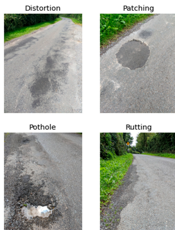
Figure 6. Examples of defects observed from the designated road segment.
