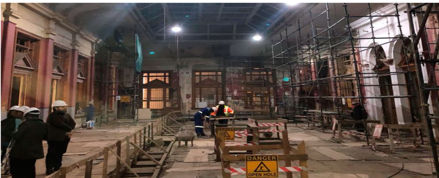
Figure 2. The main hall of the RSPO under reconstruction in 2018. Source: Steven Sack.
