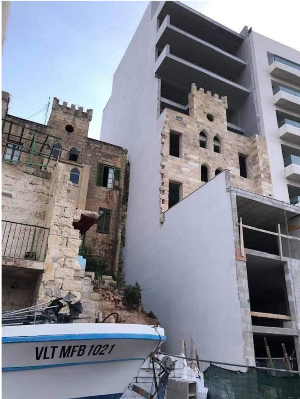
FIGURE 18 CONSTRUCTION AT SPINOLA BAY, ST JULIAN'S. PHOTOGRAPH: MARK ZAMMIT CORDINA(TIMES OF MALTA)
