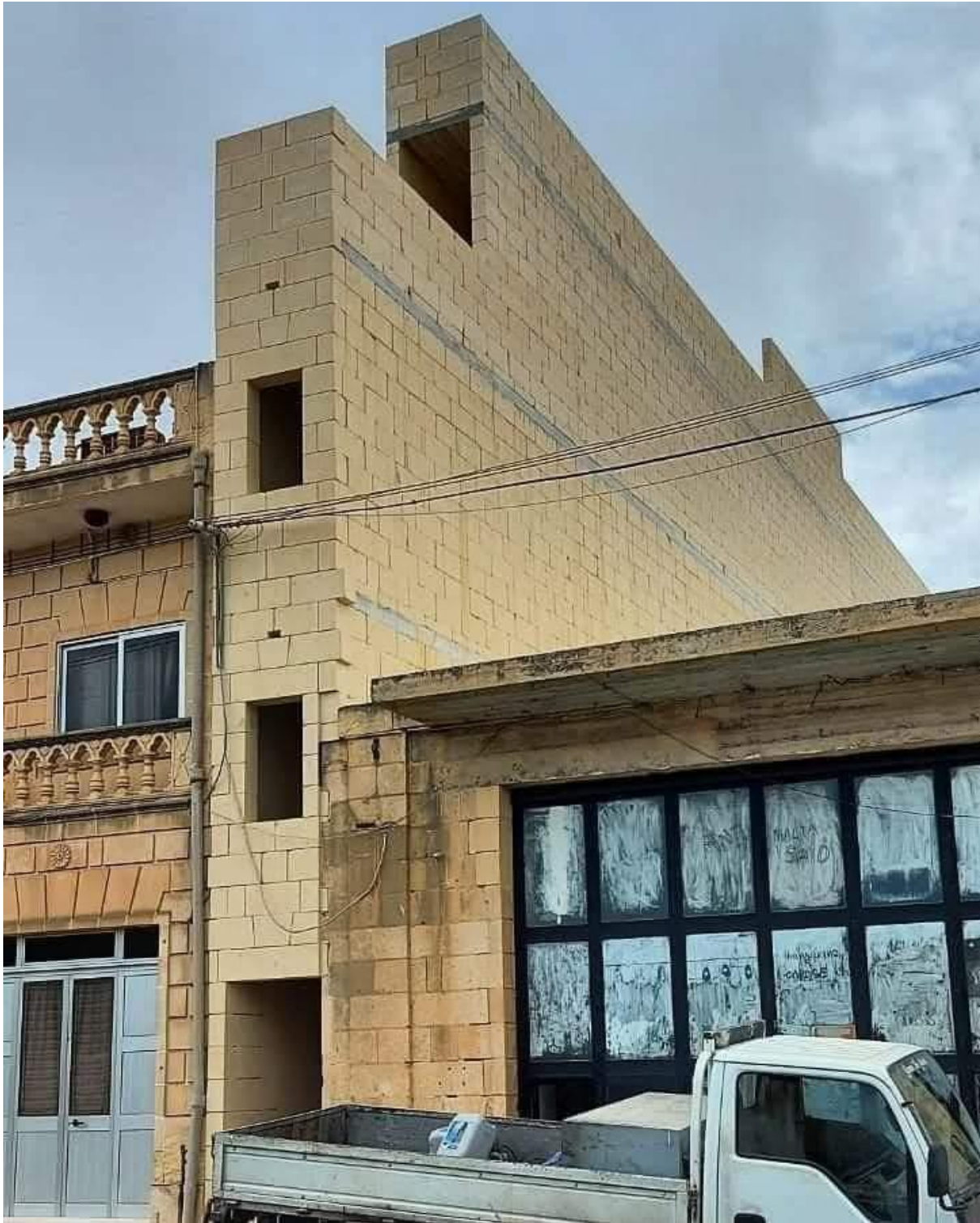
FIGURE 28 MALTA, THE BUILDING CURRENTLY UNDER CONSTRUCTION AT THE CENTRE OF THE IMAGE MAY BE UNDERSTOOD AS PART OF A BROADER PATTERN OF RECENT DEVELOPMENT THAT RAISES QUESTIONS OF BOTH AESTHETIC JUDGMENT AND ETHICAL RESPONSIBILITY. ITS NOTABLY NARROW FORM, COMBINED WITH ITS SCALE AND PLACEMENT, APPEARS TO CONTRIBUTE LITTLE TO A MEANINGFUL SENSE OF DWELLING OR SPATIAL GENEROSITY, INSTEAD EXEMPLIFYING A GRADUAL PROCESS OF VISUAL AND CONTEXTUAL DEGRADATION THAT MAY BE DESCRIBED AS TURPIFICATION.
