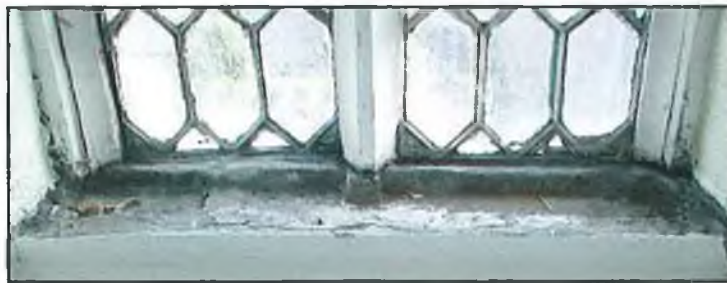
FIG. 9.10 The base of the windows is also medieval and grooves for glass are present.
