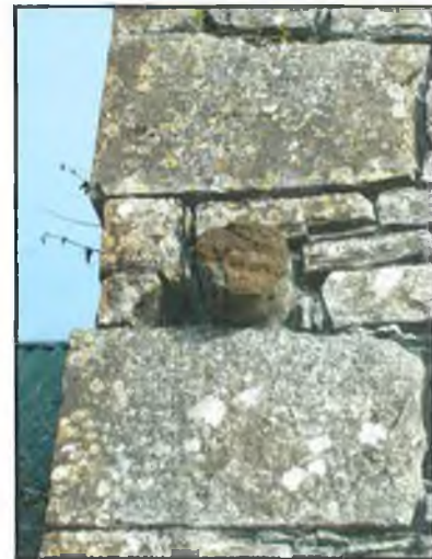
FIG. 9.25 Eroded stone head.
