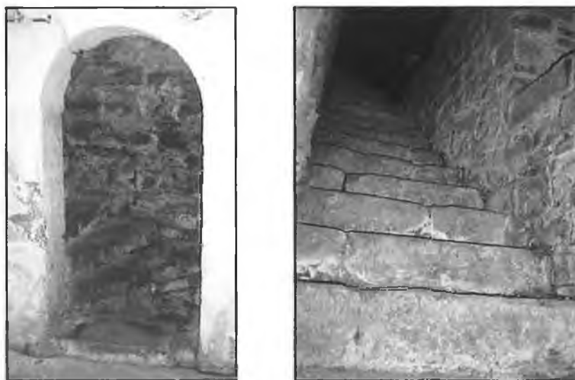
FIGS 9.3-4 One of two flights of stairs leading from basement to ground floor.
