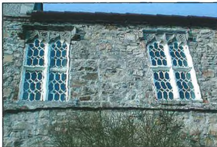
FIG. 9.8 Medieval window heads and hood-moulds of probable fifteenth-century date were reused in the construction of several windows at Talbot’s Castle. These two are on second floor level on the south façade.
