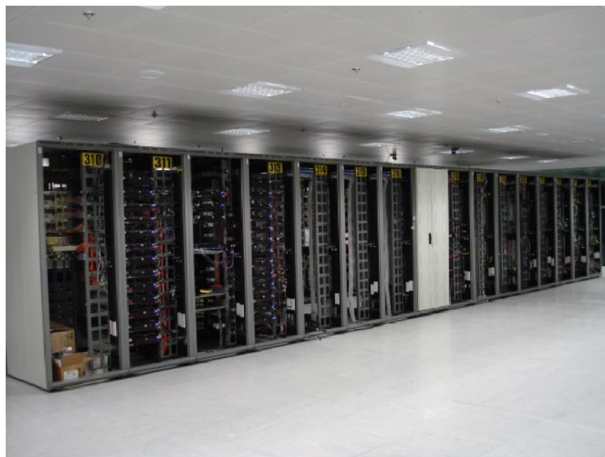
Figure 3.2. A row of server cabinets in the secure facility where the ERC Server is hosted.
