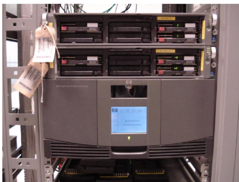
Figure 3.3. The ERC Server's high-capacity tape library used for data back-ups.
