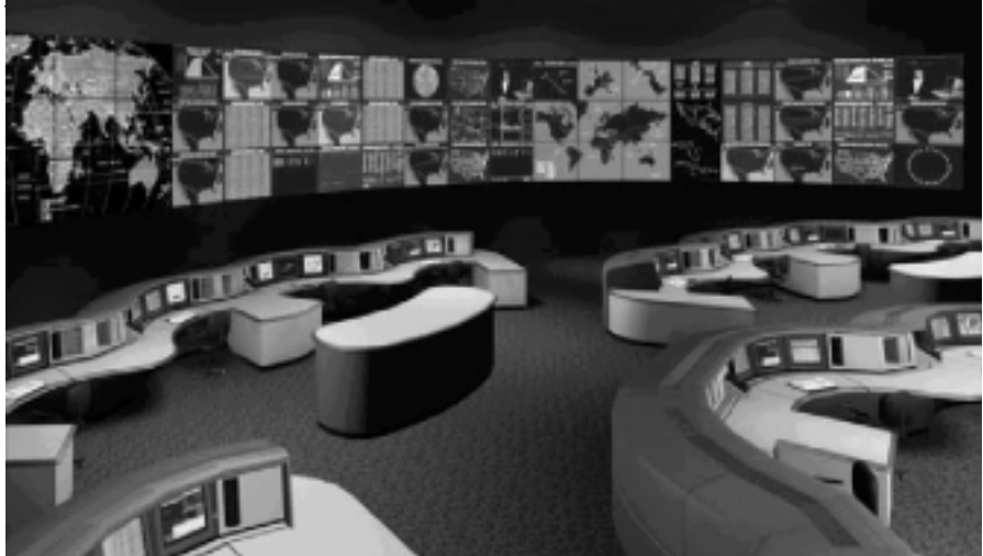
Figure 1 View of AT&T's Large NOC with Large Wall Displays Showing Network Maps
