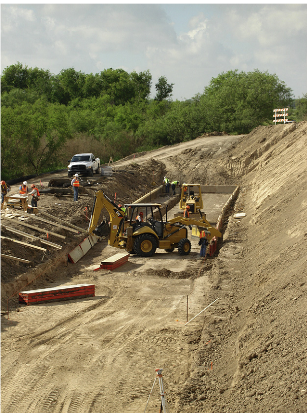
Fig. 2. Witnessing levee border wall construction at Monterrey Banco National Wildlife Refuge, 2008. Photo courtesy of Wayne Bartholomew.
